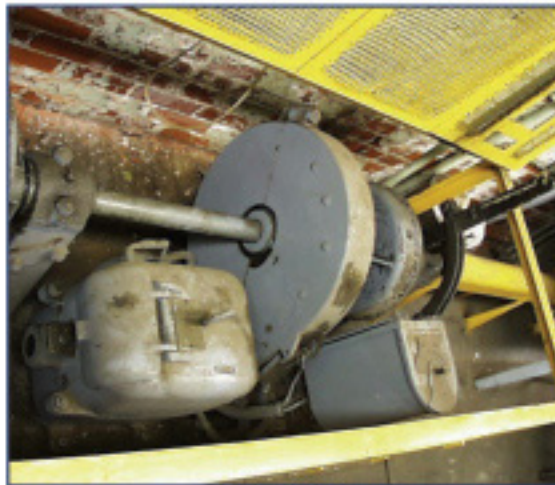
Original DC Drive System
